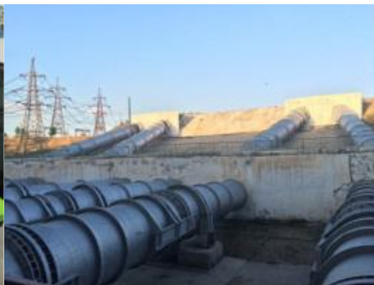
Amu-Bukhara Irrigation System
